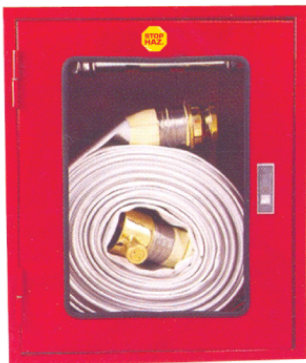
● Fire Hose Cabinet
